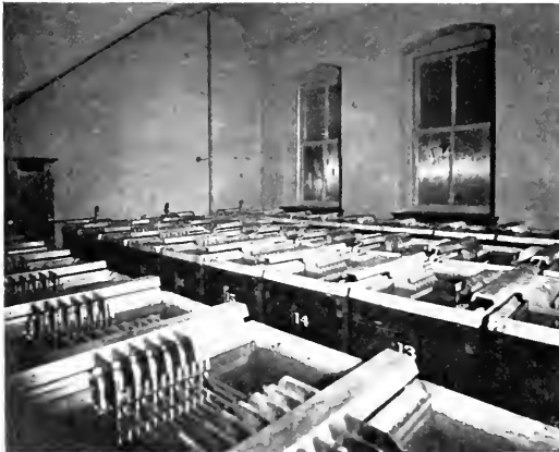
FIG. 4.—BATTERY PLANT IN MAIN EXCHANGE.
